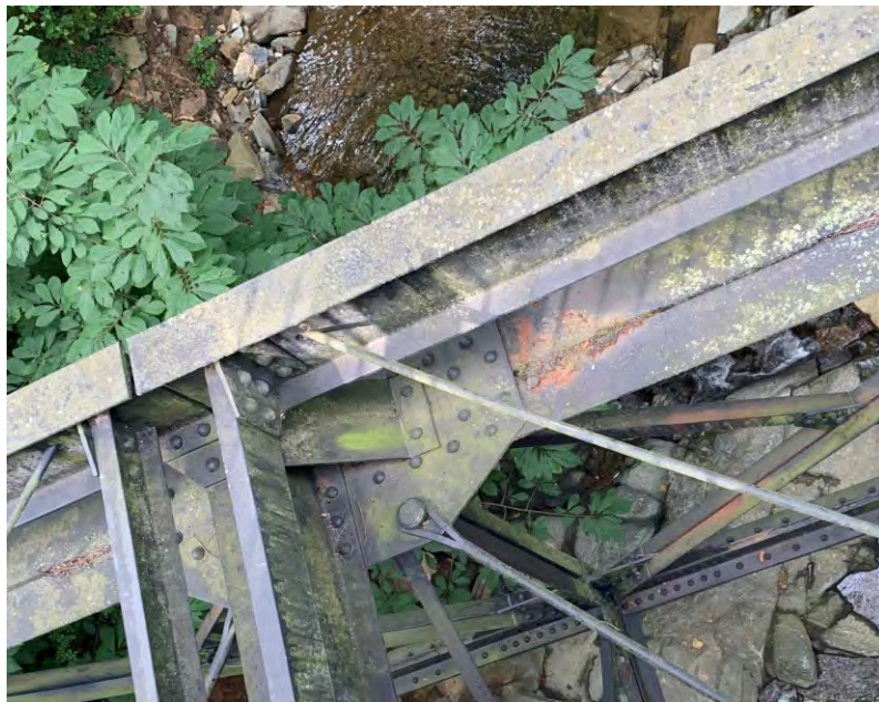
Figure 16: New Corrosion at the Rehabilitated Glen Echo Trolley Bridge (August 2019)
