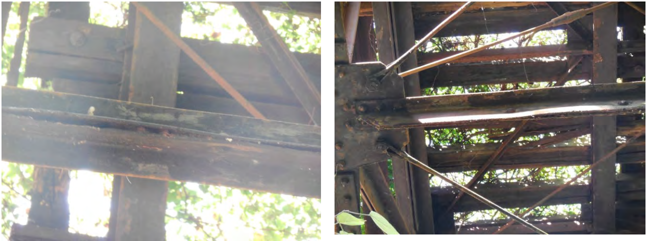
Figure 5.11: Rusting between Double Angles
