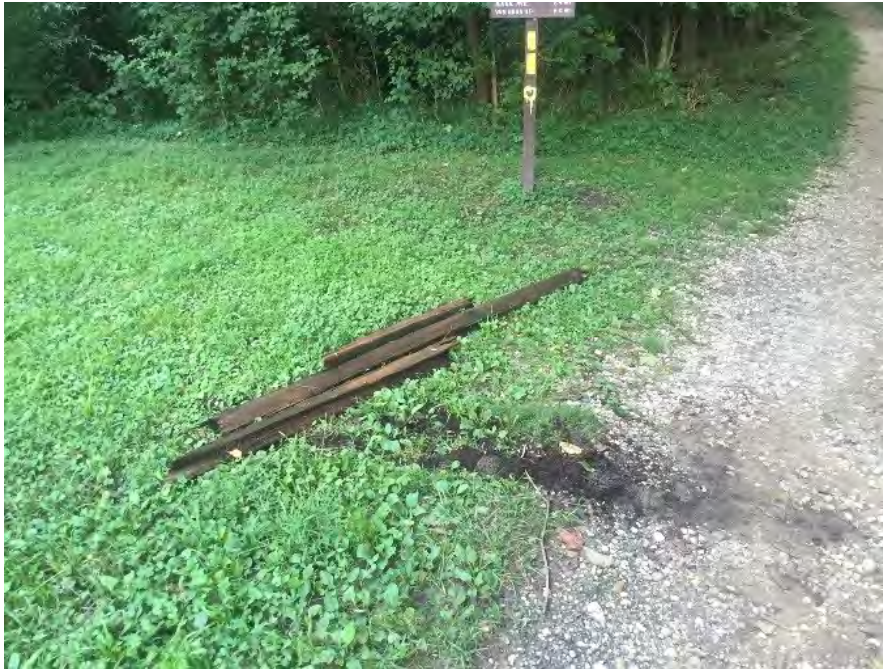
Figure 1.7: Fallen rail tie beneath the bridge (August 2, 2016)
